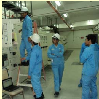
PQ Monitor Installation at Huntsman Tioxide, a petrochemical manufacturer of paint pigments, Teluk Kalung, Terengganu. In the picture are Dr. Pauzi and Mr. Lutfi, CEES engineer.
