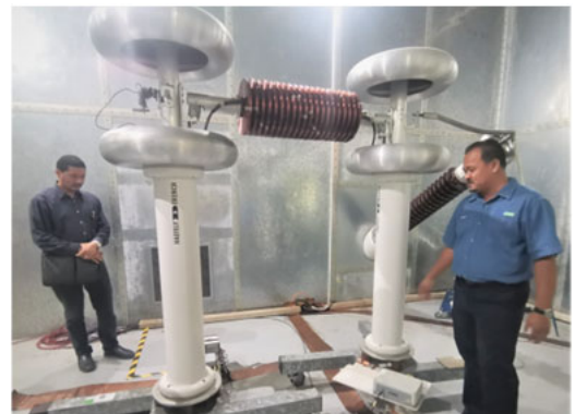
TNBR's representative (right) explaining about the facility.
