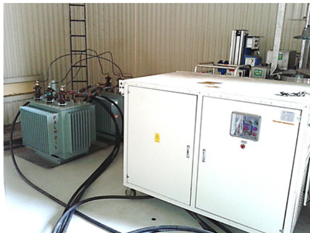
Picture of 100kVA palm-based power transformer with load bank at IVAT, under research collaboration with MPOB and Tenaga Nasional Berhad Research.
