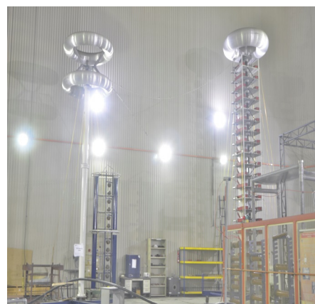
2 MV impulse generator.
