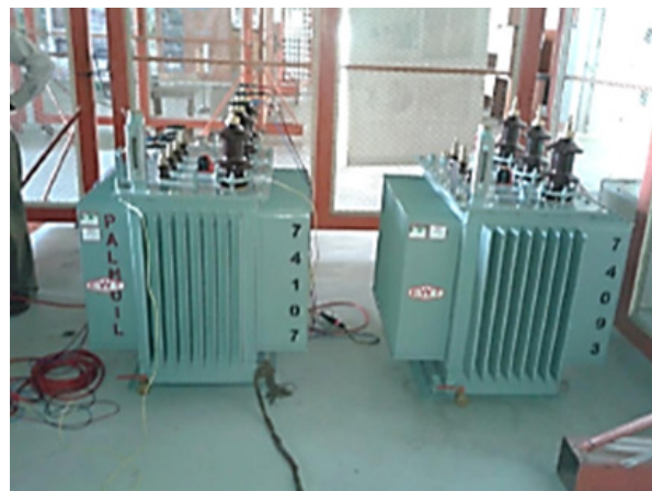
Picture of 100kVA palm-based power transformer and mineral oil-based power transformers at IVAT laboratory, under research collaboration with MPOB.
