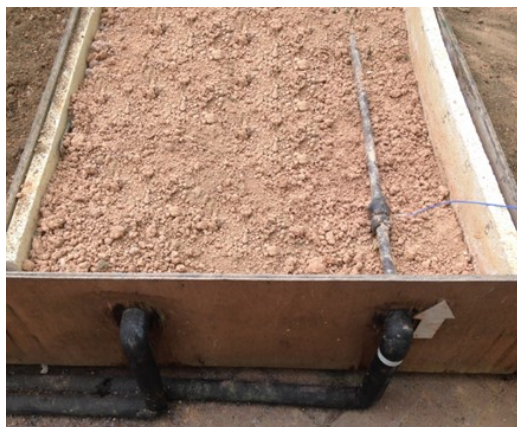
Cooled soil plot with embedded pipes
