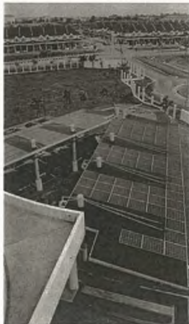
Monocrystalline PV modules (27kWp) on the carpark roof
