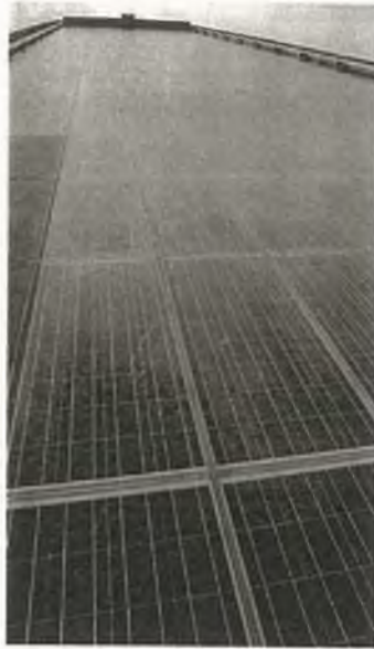
Polycrystalline modules (47.28kWp) on the main roof
