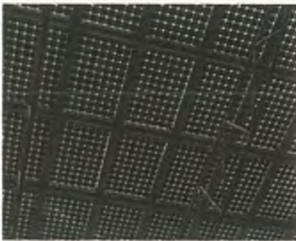
Glass semi-transparent PV modules (11.64kWp)
