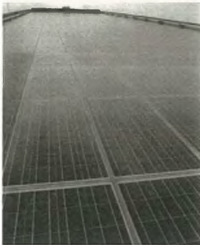
Polycrystalline modules (47.28kWp) on the main roof
